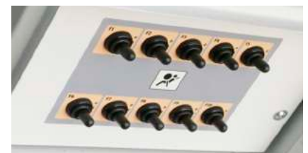
Fault switch box
