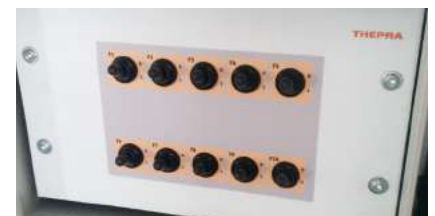
Fault switch box
